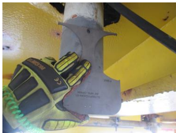
Marking on the pipe
